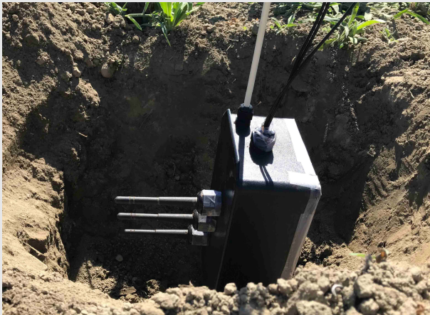
Waterproof box holding the RX antenna array
